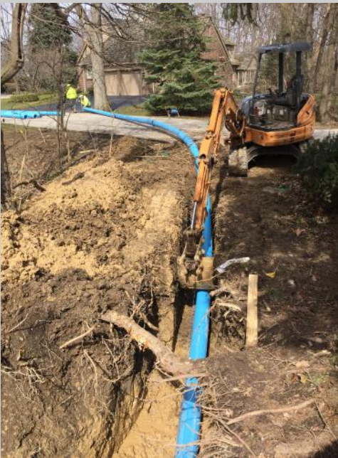
Above: Crews from Speer Bros. Inc. install the main water line at The Hamlet in Perrysburg Township. The waterline replacement project wrapped up in late May, but restoration will continue through June.
