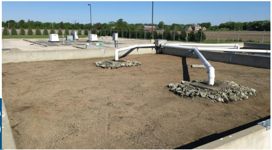
Above: Photograph of the sand filter at the Williamsburg-On-The-River package plant taken by District wastewater operator Jeff Kramer. Kramer's photographs, including the one above, are featured in the Ohio Water Environment Association's 2019 calendar.
