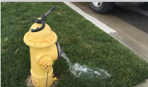
Above: District crews are in the process of flushing and painting the over 3,800 hydrants around The District.
