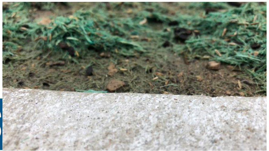
Pictured above: New sidewalk installed and grass seed planted in Rossford. We appreciate everyone's patience as we landscape this fall.
