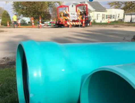
Above: Sewer work on Scott Street in McComb. We thank the community for your patience as we continue to make improvements to the water & sewer system in McComb.
