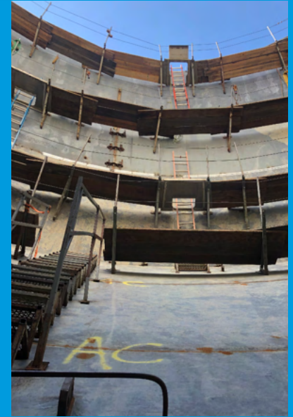
Above: A unique view from inside the water storage tank in Lake Township.
