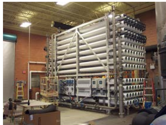
City of Bowling Green Water Treatment Plant
