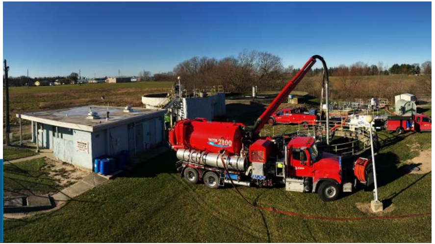
Above: Maintenance crews winterize the McComb wastewater treatment plant. The District continues to make low-cost improvements to the 70 year-old plant. The District hopes to start construction of a new plant this year. For more on this project, see Page 2.
